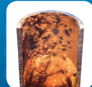
Galvanised pipe heavily corroded
