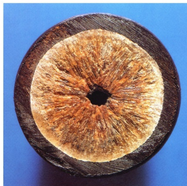
Copper pipe - heavily scaled
