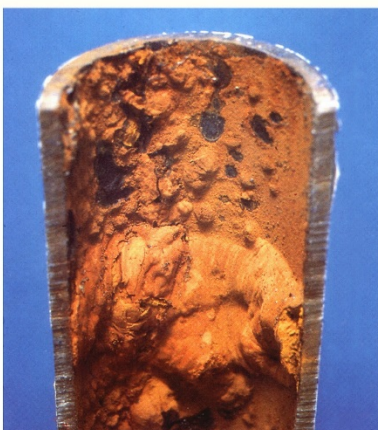
Galvanized pipe heavily corroded
