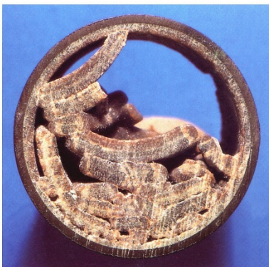
Copper pipe with scale plug
