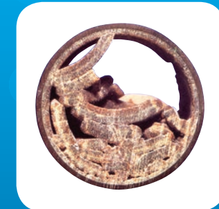
Copper pipe with scale plug
