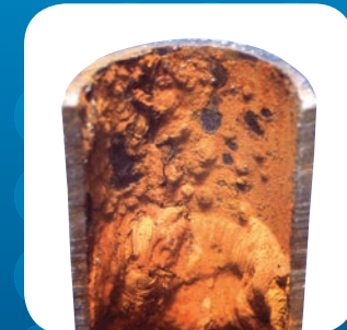
Galvanised pipe heavily corroded
