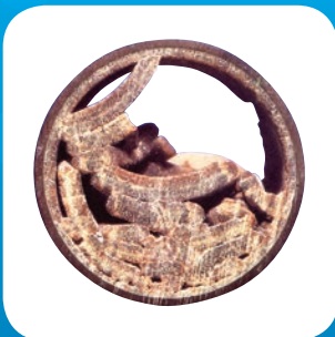
Copper pipe with scale plug
