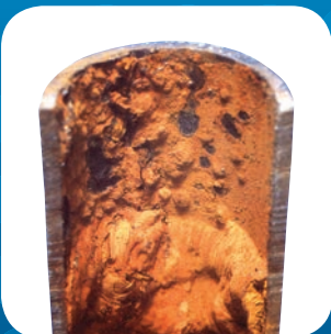
Galvanised pipe heavily corroded
