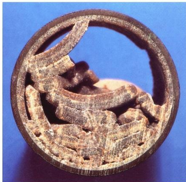
Copper pipe with scale plug
