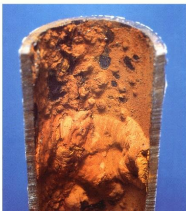
Galvanized pipe heavily corroded
